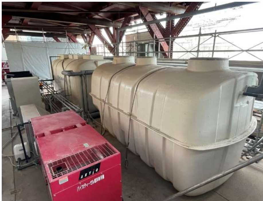
AQUAMAKE Installation Status
