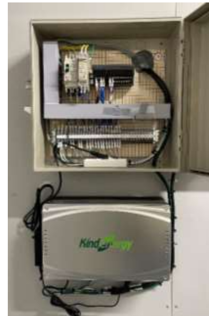
K-BOX and control panel installed in the pavilion
