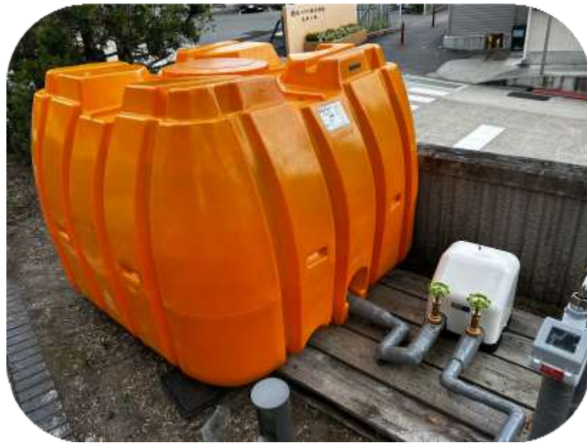
Transporting surplus water from the site to the factory
