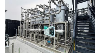
CO 2 recovery equipment
