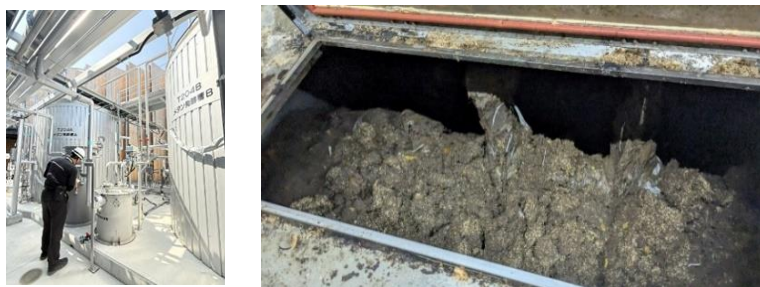
Figure 3-2-42 Biogas equipment at the Japan Pavilion (left), composting machine in the main stockyard (right) Source: Japan Pavilion Official X ( https://x.com/japanpavilion_j/status/1942524100779663459/photo/2 )
